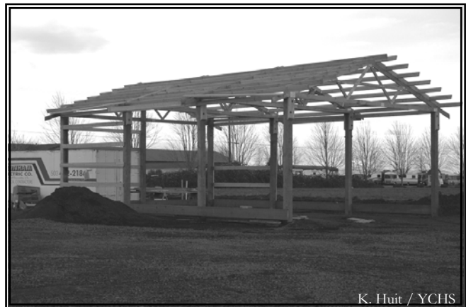
When complete, the Sawmill Building, constructed by volunteers, will house the operational 1910 Deloach Sawmill.
